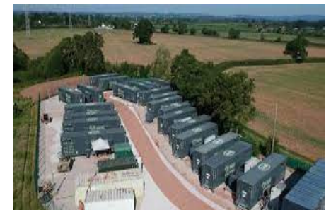
S Somerset battery storage
