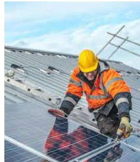
Bristol Energy Coop solar roofs
