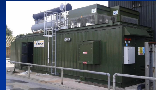
CHP facility in Belfast CC / Queen's Uni
